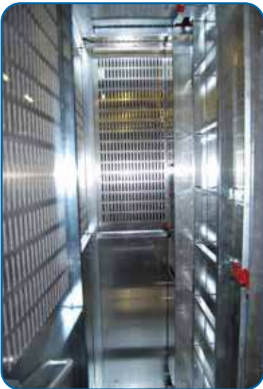
Interior de cabina Interior of the cabin
