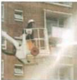
Water jet and fog curtain.
