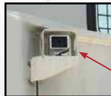
Integrated air conditioning
