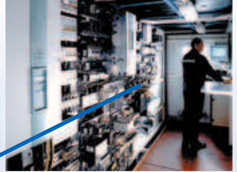
Air-conditioned electric compartment
