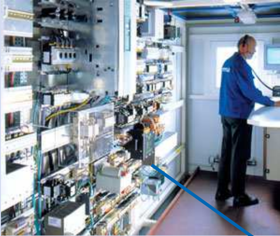
Air-conditioned electrics compartment
